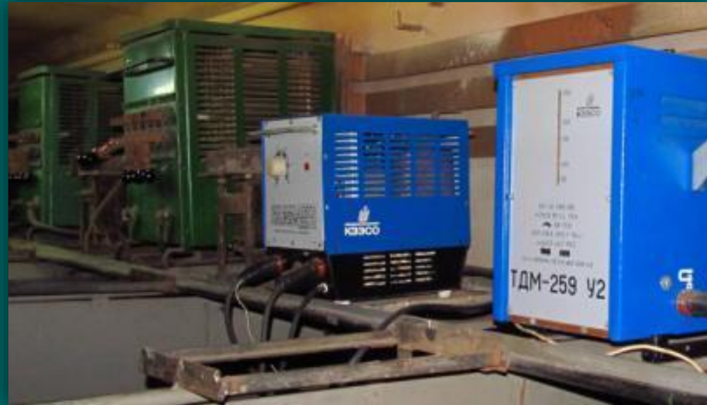
welding power supplies
